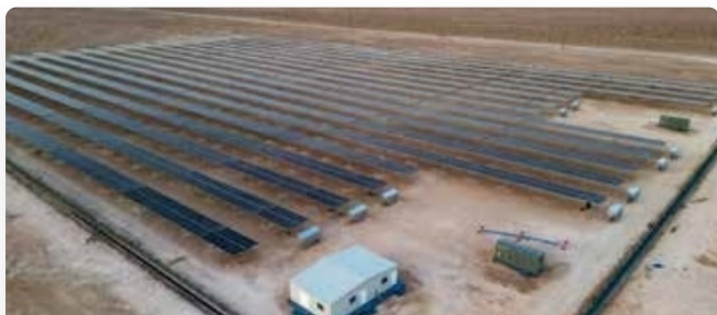
Single Axis Tracking Solar System, Thumeraith — 7 MWp
