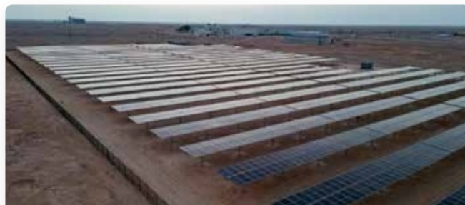
Oman Cements — On-Grid Solar Power System (100 kW), 2019
